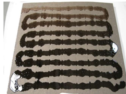
Freshly applied beads of XR Stick on mechanically attached Polyisocyanurate insulation board @ 4" o.c.
