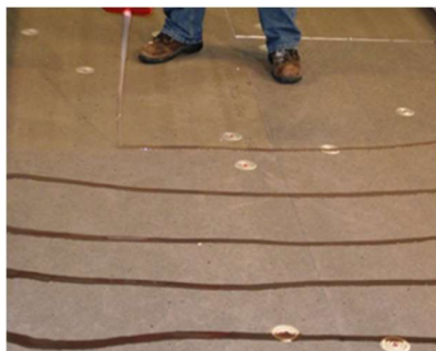
Bead application of XR Stick in cartridge on mechanically attached Polyisocyanurate insulation board @ 12" o.c.
